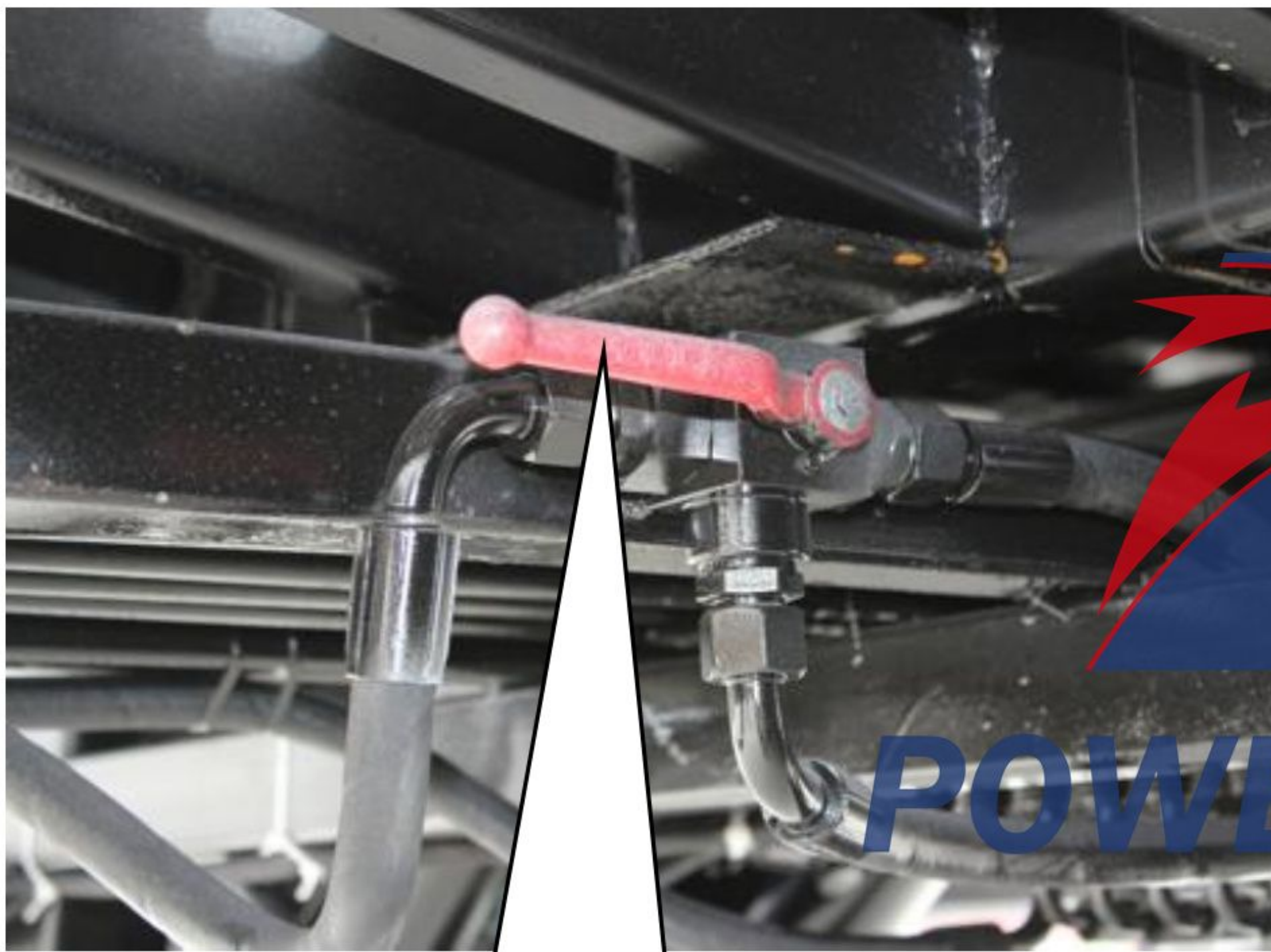
Figure 1: Red Switch parallel with platform
